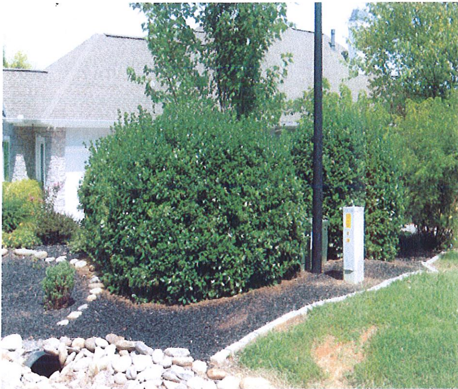
(Example of Obstructive Underground Electric Transformer)
